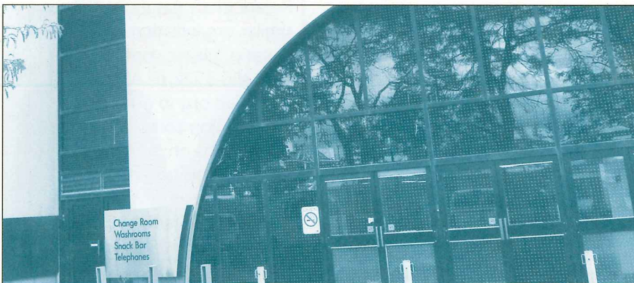
Feather Friendly® "symmetry pattern" applied to the southwest entrance of the Scarborough Civic Centre.
